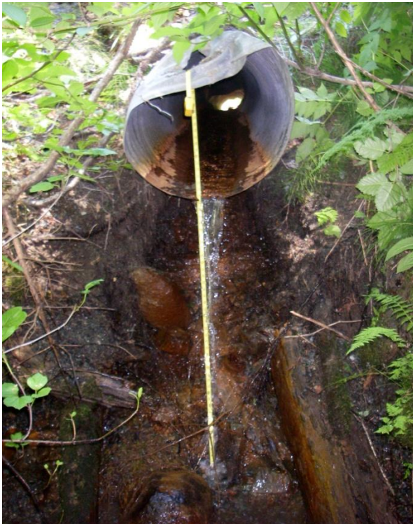
Culvert Perch before replacement
